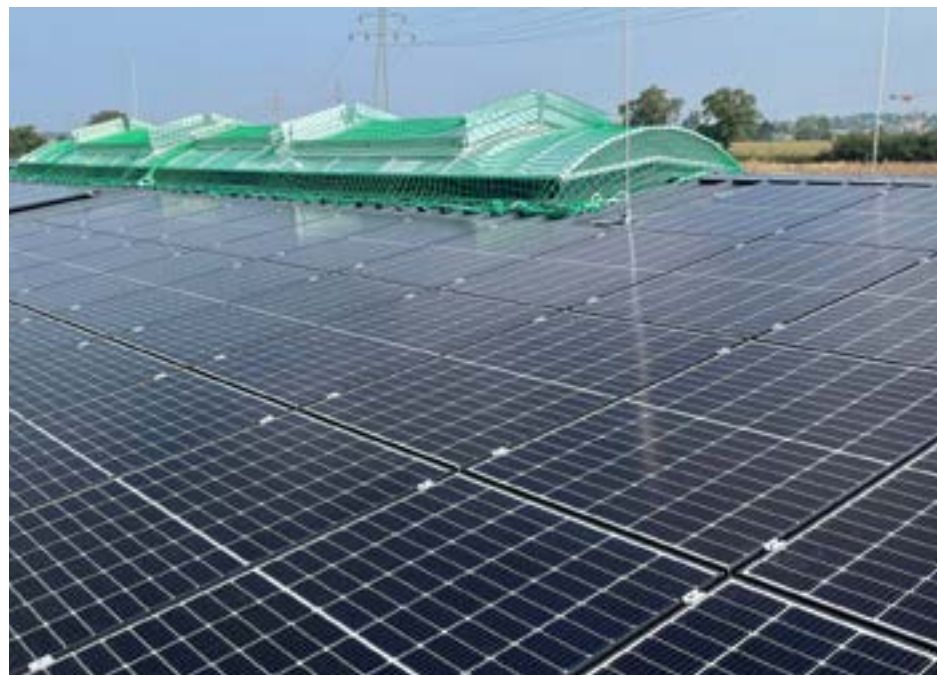
Photovoltaik Hall de stockage
